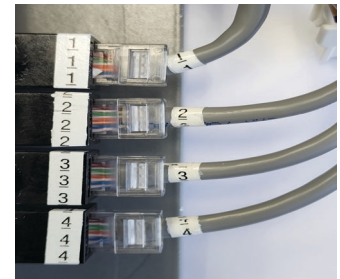
RJ45 coupler on remote display connected to RJ45 from surge enclosure
